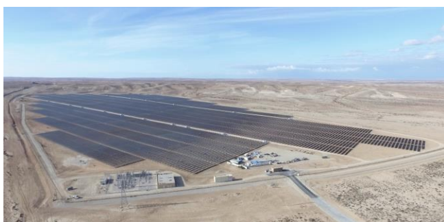
Caption: Ashalim solar power plant is located in the Israeli Negev Desert. Picture credit: BELECTRIC
